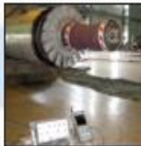
RSO on 250 MW TG Rotor Winding
