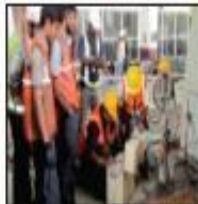
DC HV Test on Winding
