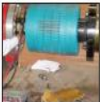
BLE Rectifier Assembly Checks
