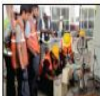
DC HV Test on Winding
